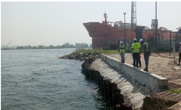
Project Site: LADOL, Lagos Free Zone Remedial Works for the Repair of Failed Sheet Pile at LADOL.
